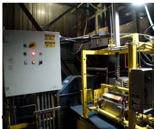
OXEA installed at a bypass in the Conemaugh power - plant (2013).
